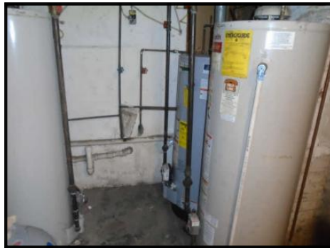
3 HOT WATER HEATERS
