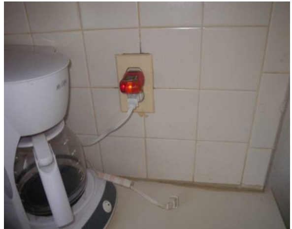
No GFCI reversed polarity on kitchen counter.
