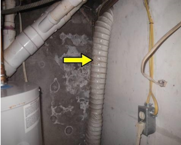
Replace plastic laundry vent for safety.
