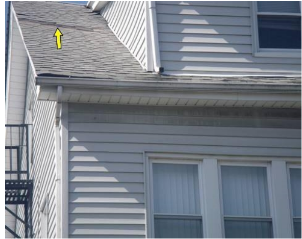
Shingles missing here.
