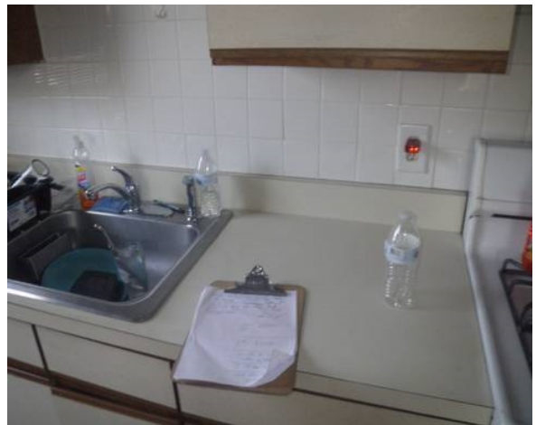
No GFCI in kitchen.
