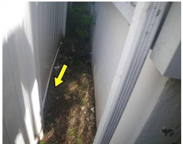
Extend discharge from sump pump further away from foundation wall.
