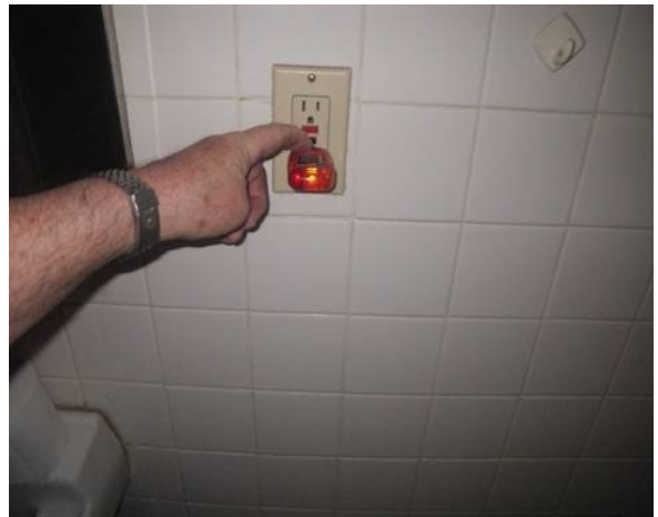
GFCI in bathroom wouldn't turn off.
