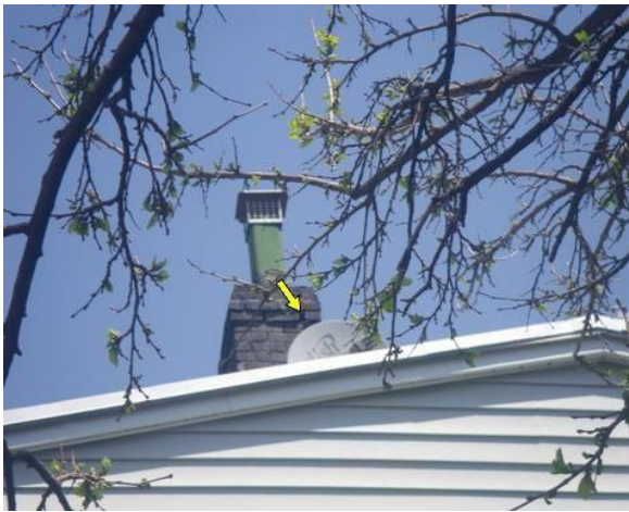
Gaps in chimney bricks can be seen from back yard.
