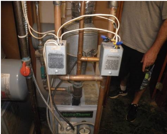
2 zones on first floor boiler.
