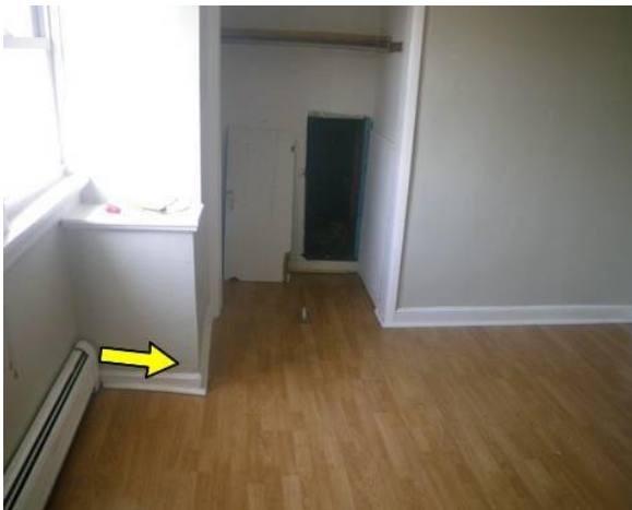
Some of flooring in top unit is uneven.
