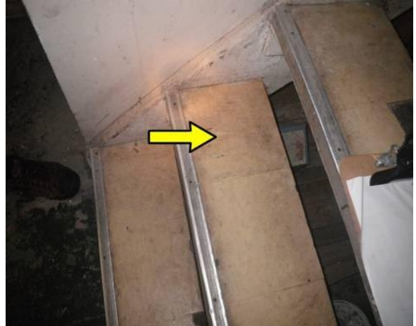
Vinyl tiles on staircase are size and age that typically contain asbestos.
