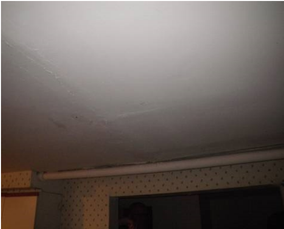
Patched cracks in basement kitchen ceiling.
