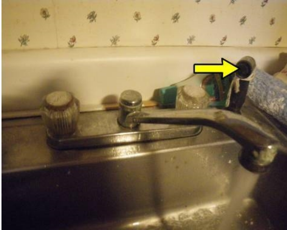
Basement kitchen hose wand is clogged.
