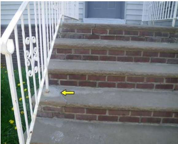
Cracked stone on lower step.
