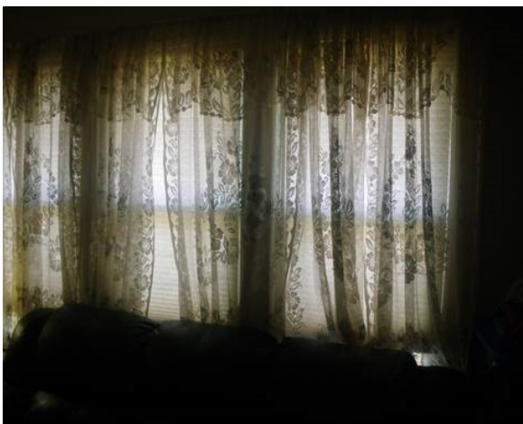
First floor front living room windows slam down if released.
