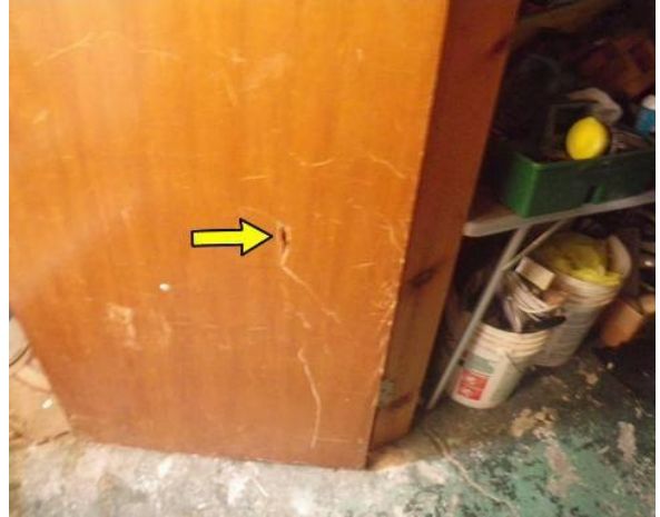
Hole in basement door.
