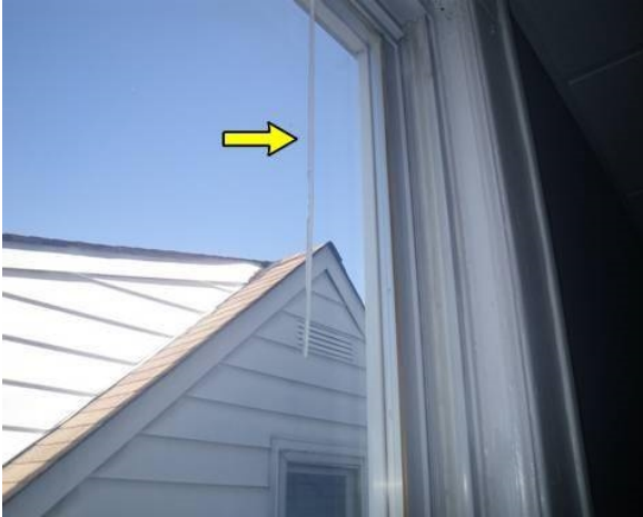
Sealing strip loose from top of side window.
