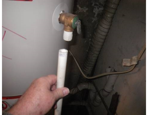
Pressure relief tube fell off hot water heater.
