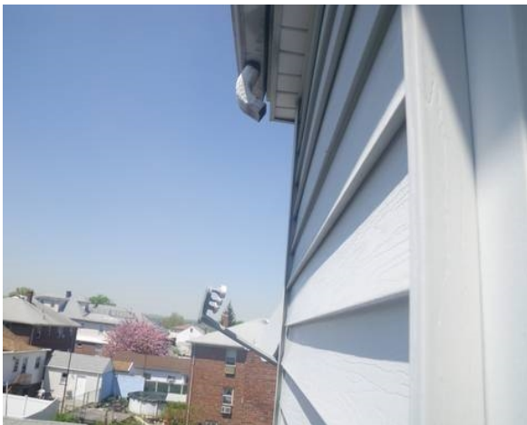
Downspout missing from top back roof.
