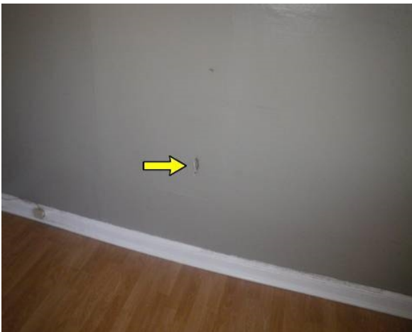
Hole in wall of top unit.
