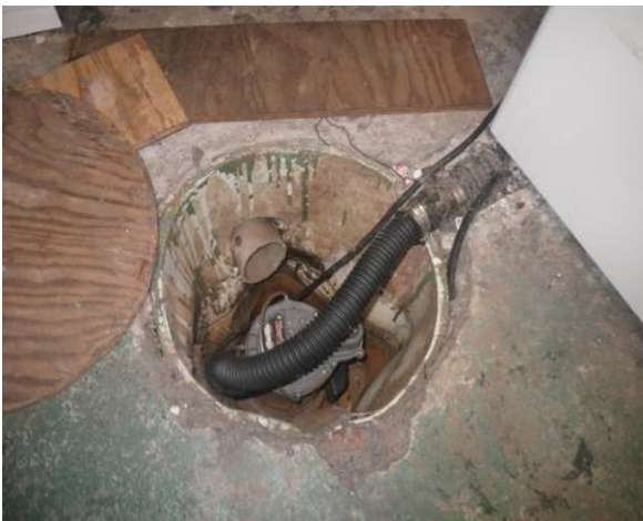
Sump pump in laundry area.
