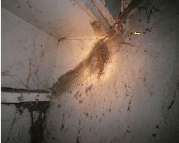
Sawdust and carpenter ant pieces under basement staircase.
