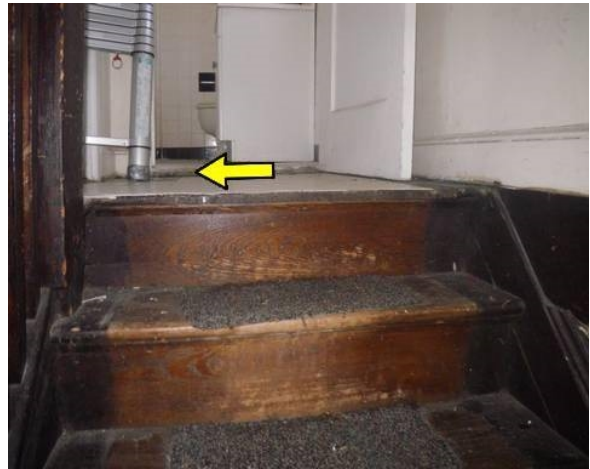
Stairway tilts towards center of building on top floor.
