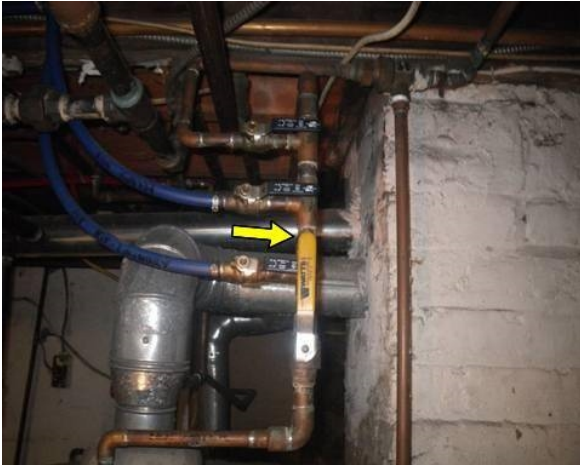
Vent for hot water heater pitches down.
