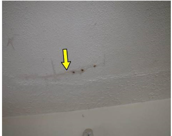
Stain on first floor ceiling and holes tested normal for moisture at time of inspection.
