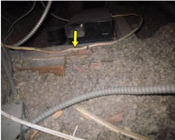
Top unit exhaust fan into attic.
