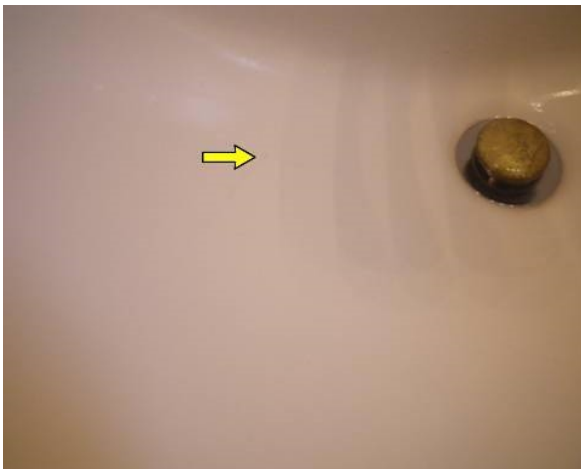
First floor vanity sink has a small crack.
