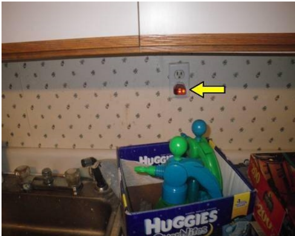
No GFCI near basement kitchen sink.
