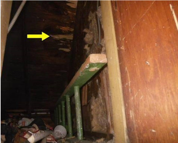
Mold-like growth in front lower attic on sheathing.
