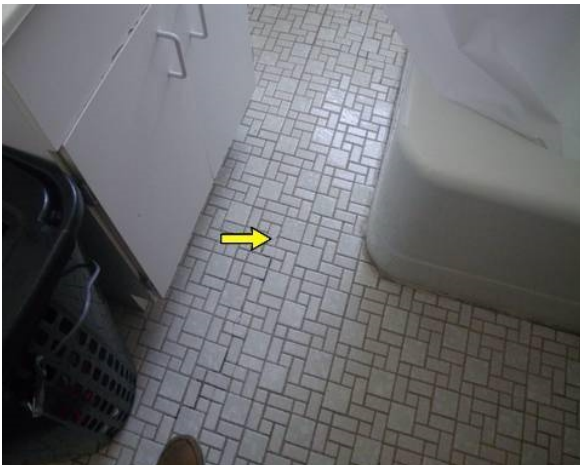
Cracked tiles here.
