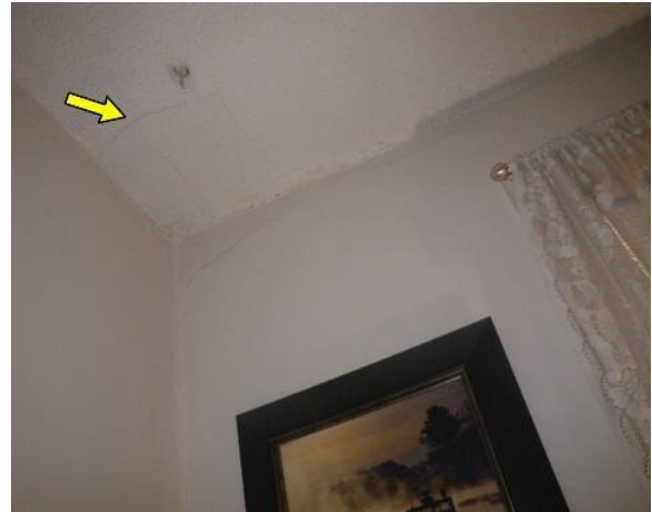
Ceiling cracks in second floor living room.
