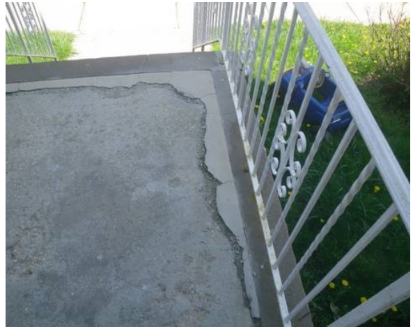
Spalled concrete on front porch deck.
