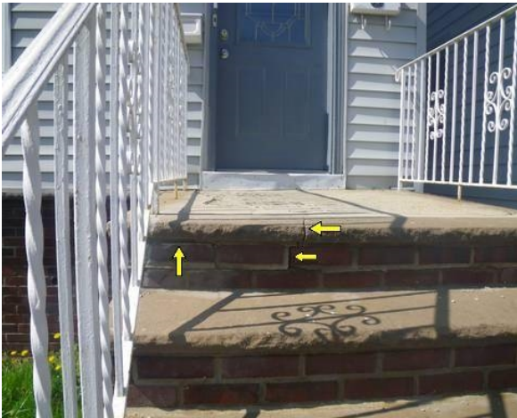
Cracks on front stairway here.
