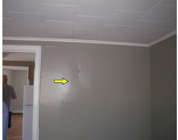
Dent in wall of top unit here.
