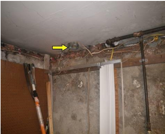
cover open electrical boxes.
