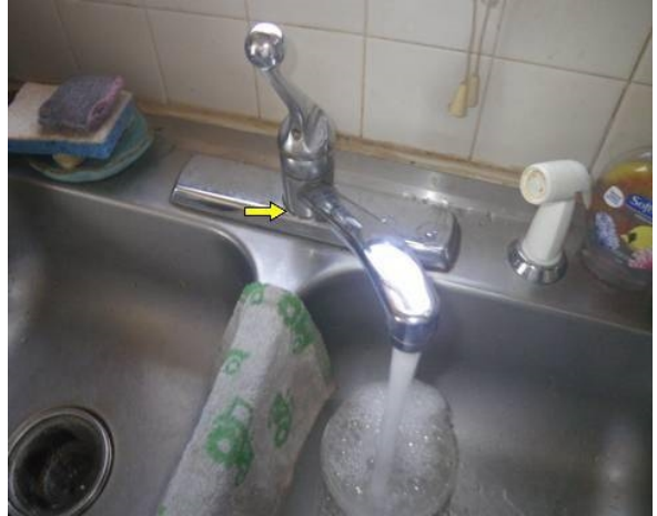
First floor faucet leaked at pivot point.
