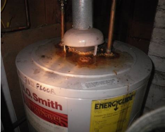
Second floor hot water heater had an active leak.
