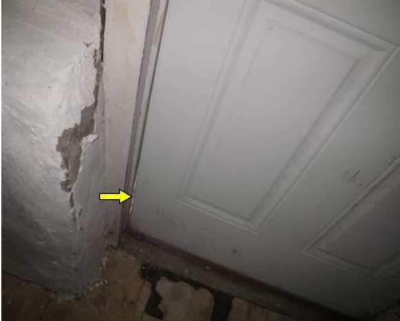
Better seal side basement door.
