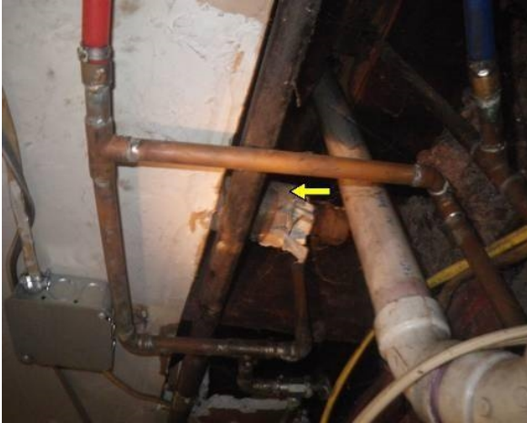
Asbestos like covering on old heating pipe.
