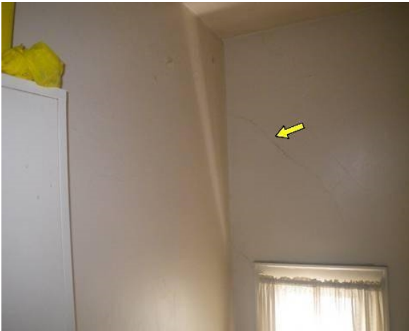
Cracks in back stairway wall.
