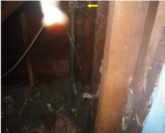
Vent stack pipe in closet has an opening on side.
